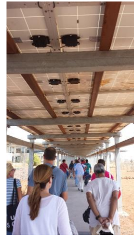
Fig. 14 Seymour Airport power plant
