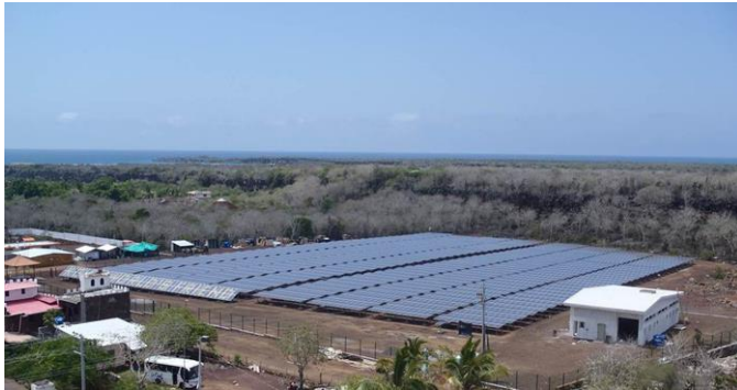
Fig. 13 Puerto Ayora solar PV power plant
