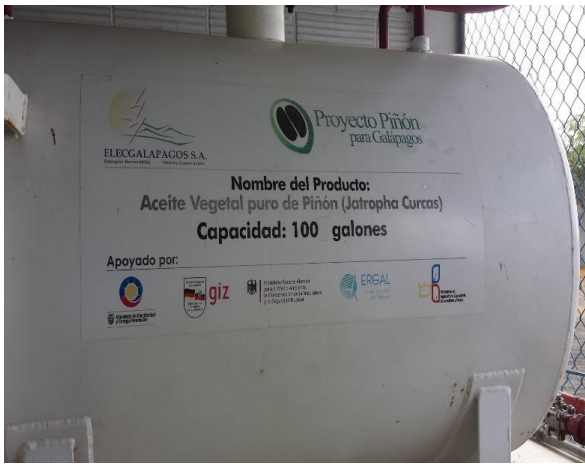
Fig. 15 Floreana biofuels storage tank
